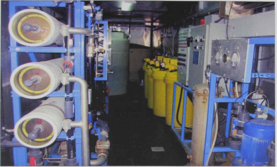
Figure B3: Mobile Desalination Plant, Al Wagan
