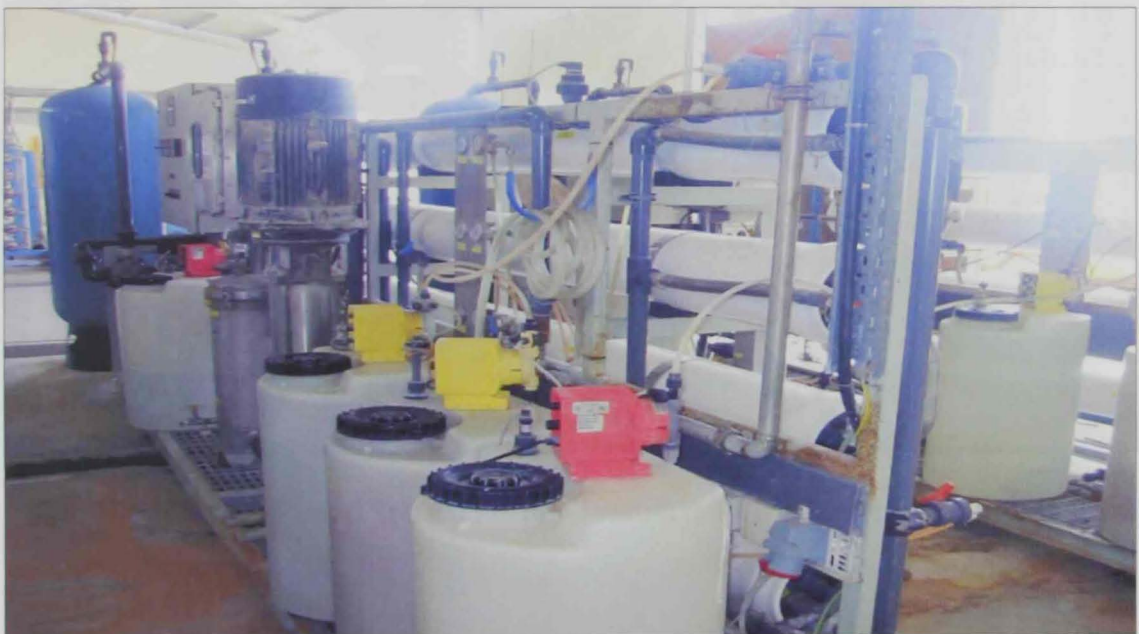
Figure B.2: Chemical used for various purposes in RO Desalination Plant, Al Wagan
