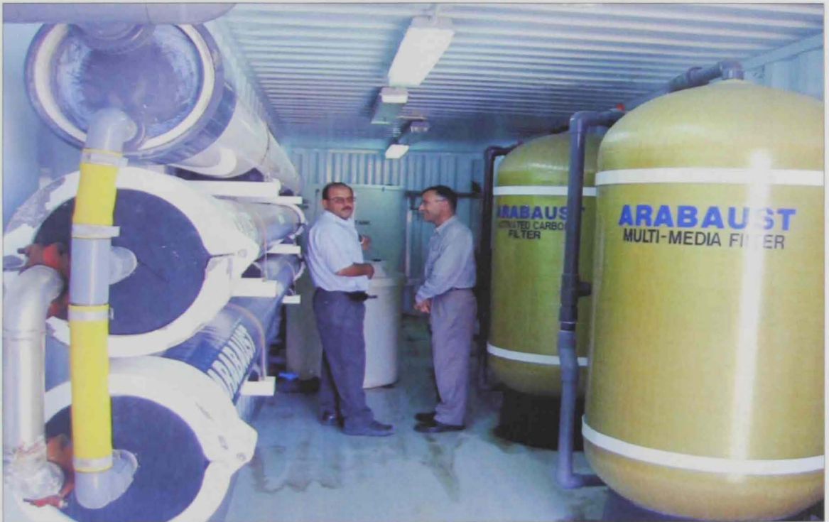
Figure B.4: Sand Filtration used for Pre-Treatment of Feed water, Mobile RO Plant
