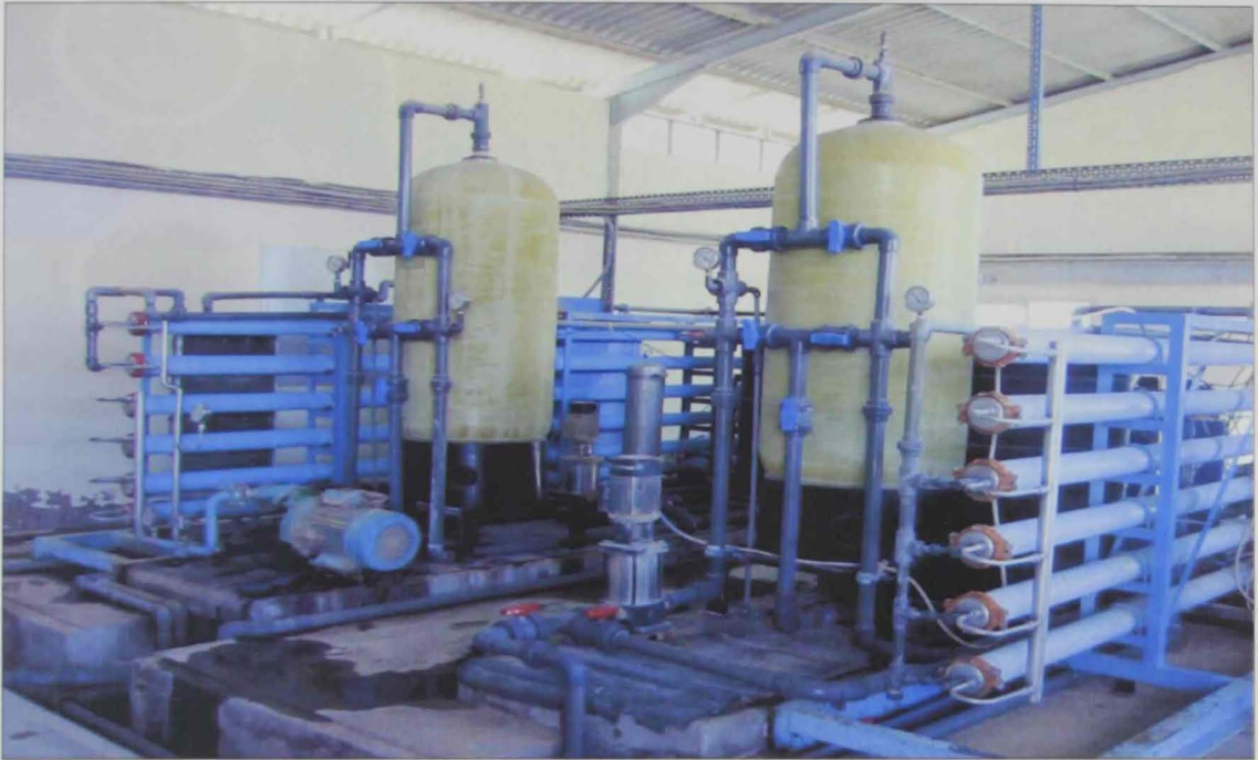
Figure B1: Al Wagan Desalination Plant
